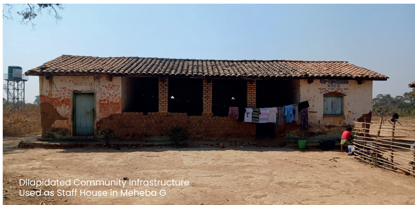
Figure 2.32: Dilapidated Community Infrastructure Used as Staff House in Meheba G
