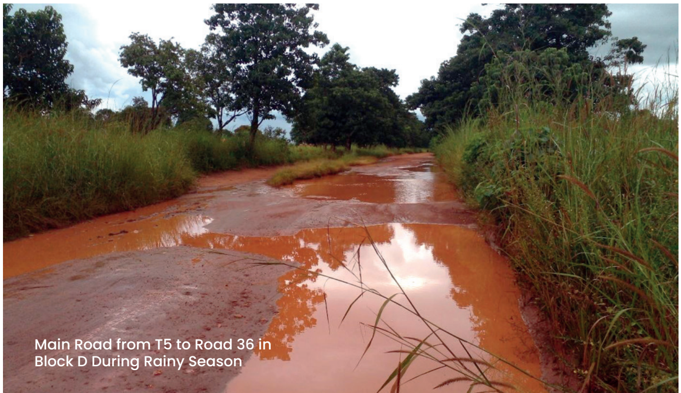
Figure 2.18: Main Road from T5 to Road 36 in Block D During Rainy Season
